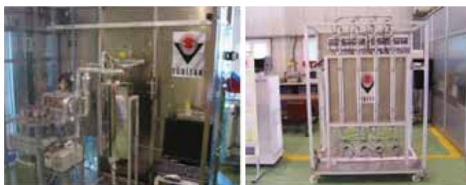
Figure 11. a) Hydrogen production (reformer) unit b) PSA unit
