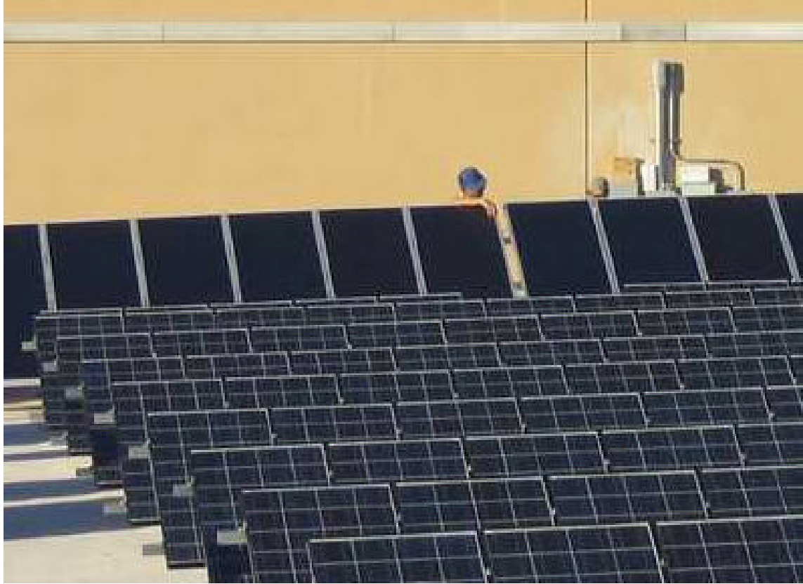
Fig. 7. Tilted Thin Film PV panels and Tilted Crystalline PV Panels
